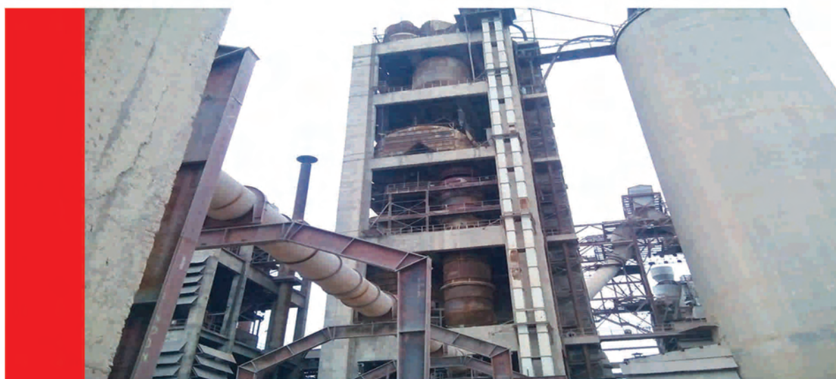
Kiln-II Preheater Rehabilitation by increasing height of Calciner, increasing Dia of Tertiary Air Duct & Downcomer Duct
